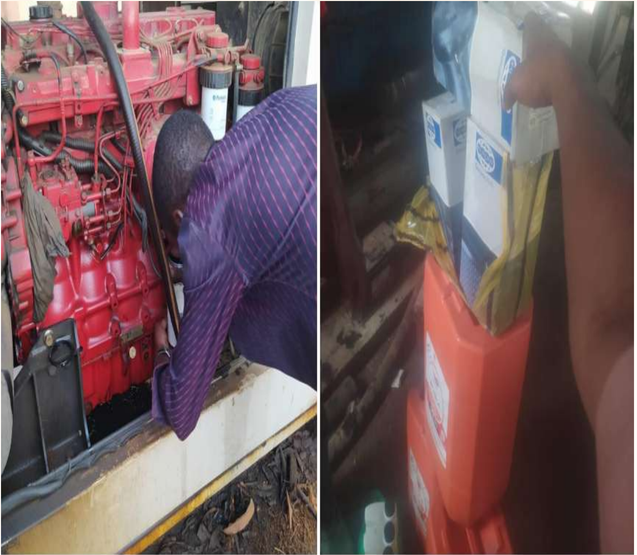
Figure (14). Routine Services of Guest House Generator at the Main Campus
