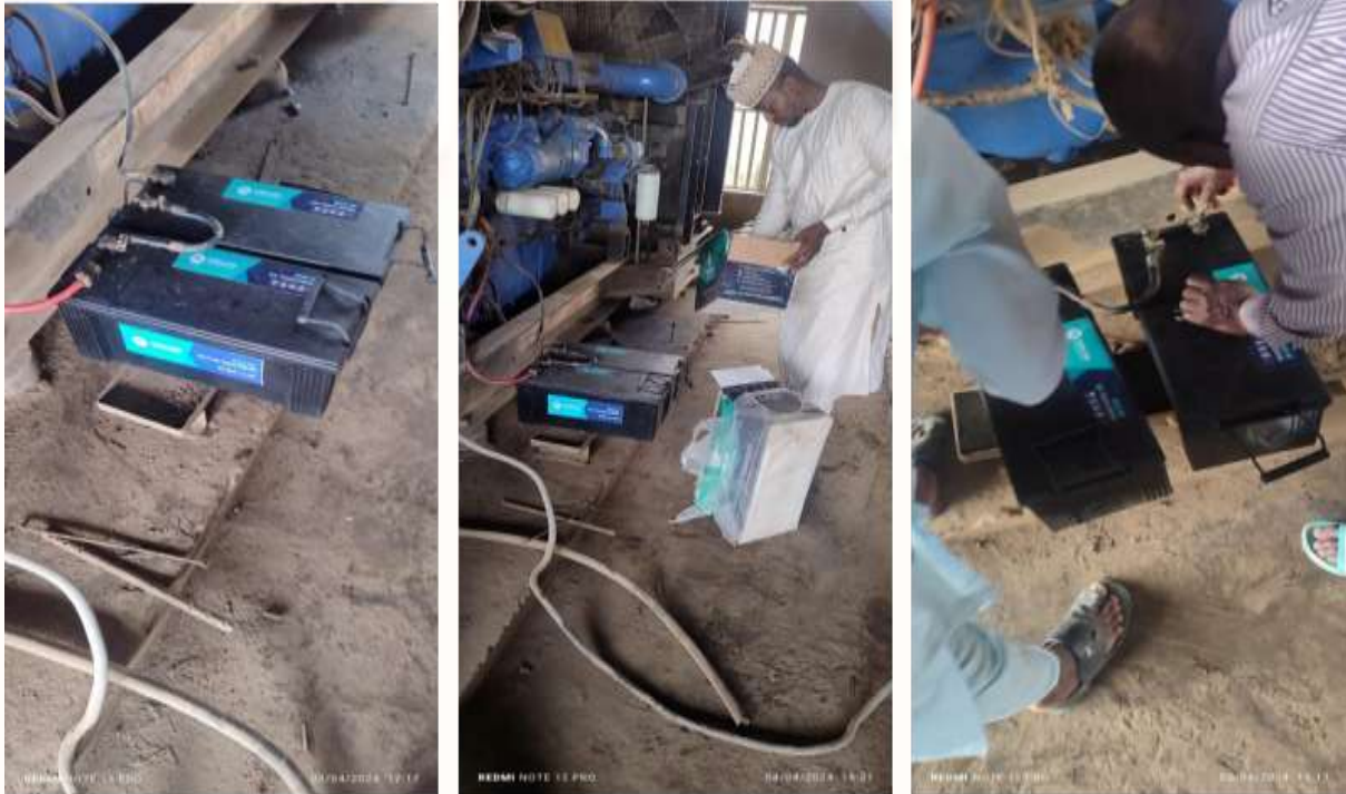
Figure (7). Purchasing and installations of 2no.s 150Ah Batteries for the set 'B' generator at the City Campus
